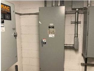
Automatic Transfer Switch - 400 Amp
