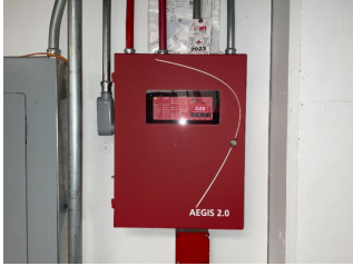
Fire Alarm System - FACP
