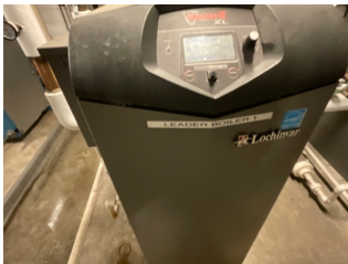
Water Heater - Gas - Comm - 700 MBH (x2)*
