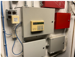
Security System - Access Control System
