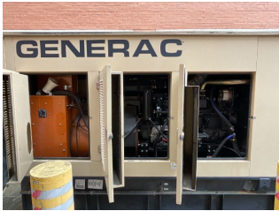
Emergency Generator - 150 kW
