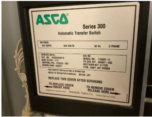
Automatic Transfer Switch - 400 Amp
