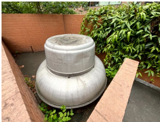
Exhaust System - General Building and Restroom
