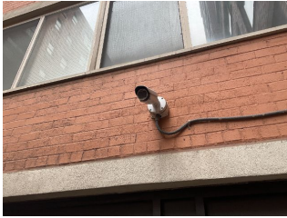
Security System - CCTV Video - Average Density - New
