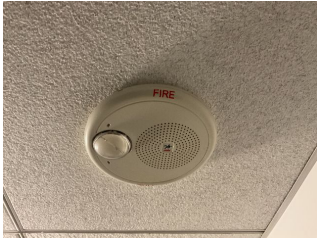
Fire Alarm System - Initiating & Alarm Devices
