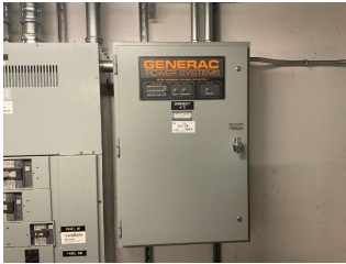
Automatic Transfer Switch - 200 Amp
