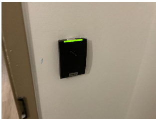
Security System - Access Control System
