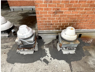
Exhaust System - General Building and Restroom
