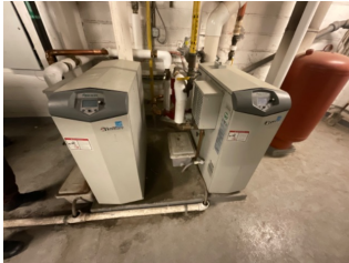
Water Heater - Gas - Comm - 700 MBH (x2)*
