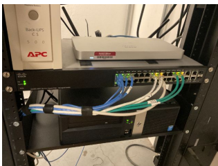
Security System - CCTV Video - Average Density - New
