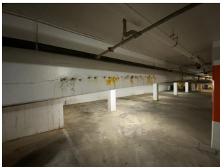
Crack along Beam
