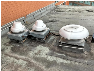
Exhaust System - General Building and Restroom
