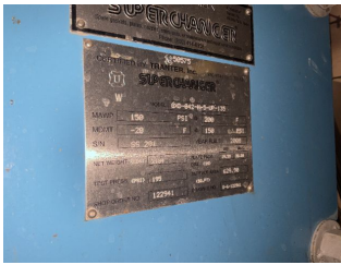
Heat Exchanger - Condenser Water
