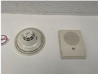
Fire Alarm System - Initiating & Alarm Devices
