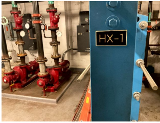
Heat Exchanger - Condenser Water
