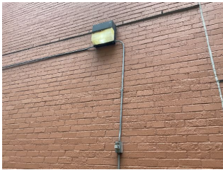
Lighting Fixtures - Exterior - HID Wall Packs
