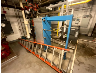
Heat Exchanger - Condenser Water
