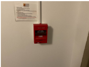
Fire Alarm System - Initiating & Alarm Devices
